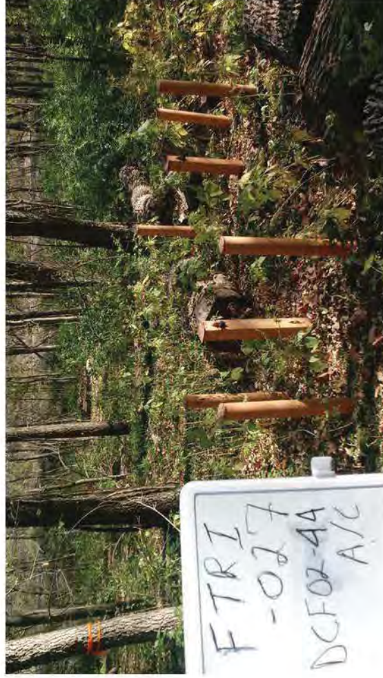
DCF02-44 A_front C_back Before Maintenance
