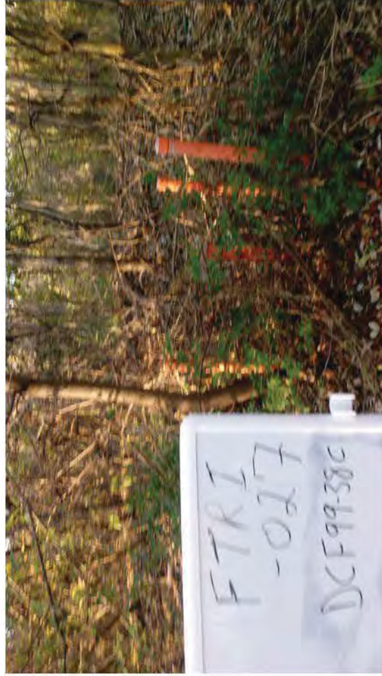
DCF99-38C Before Maintenance
