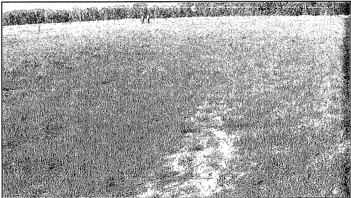
Photograph SFL2009-4 – View looking west of differential settlement/ponding in east central portion of landfill (11 May 09).
