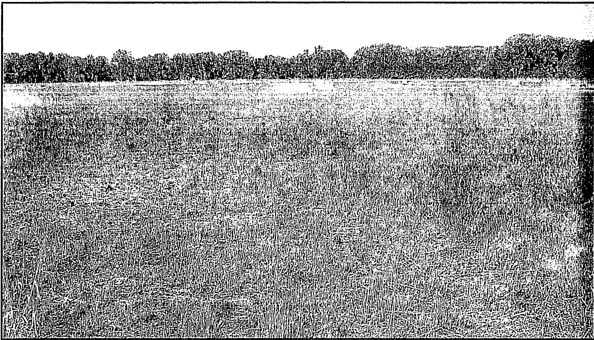
Photograph SFL2009-5 – View looking west of differential settlement in central portion of east half of landfill (11 May 09).
