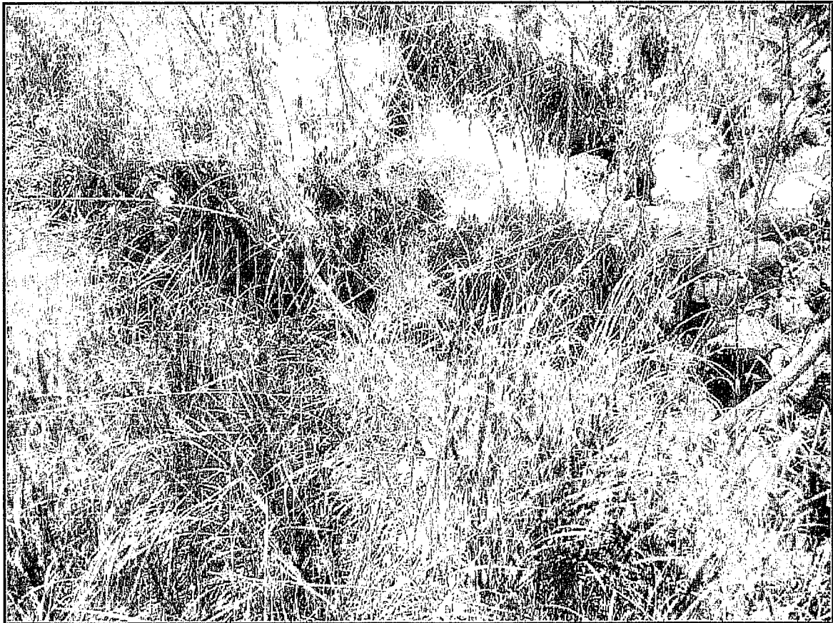
Photograph SFL2009-8 – Back cut erosion at downstream end of revetment (11 May 09).
