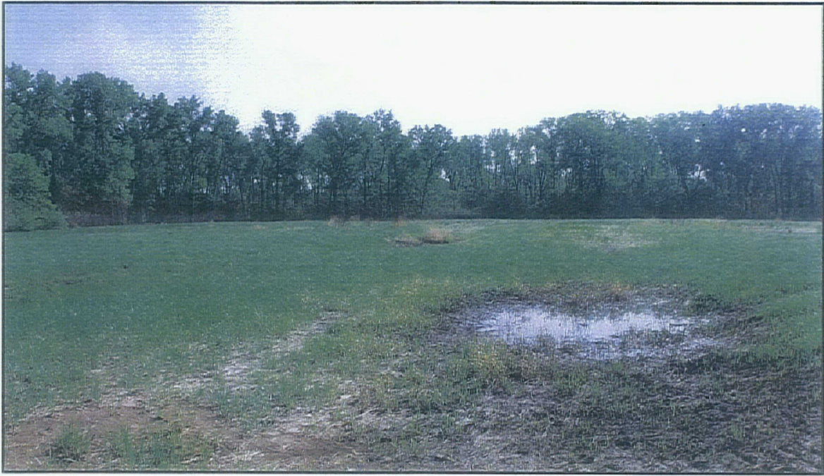
Photograph SFL2009-1 – View looking east of differential settlement/ponding in northeast quadrant of landfill (11May 09).
