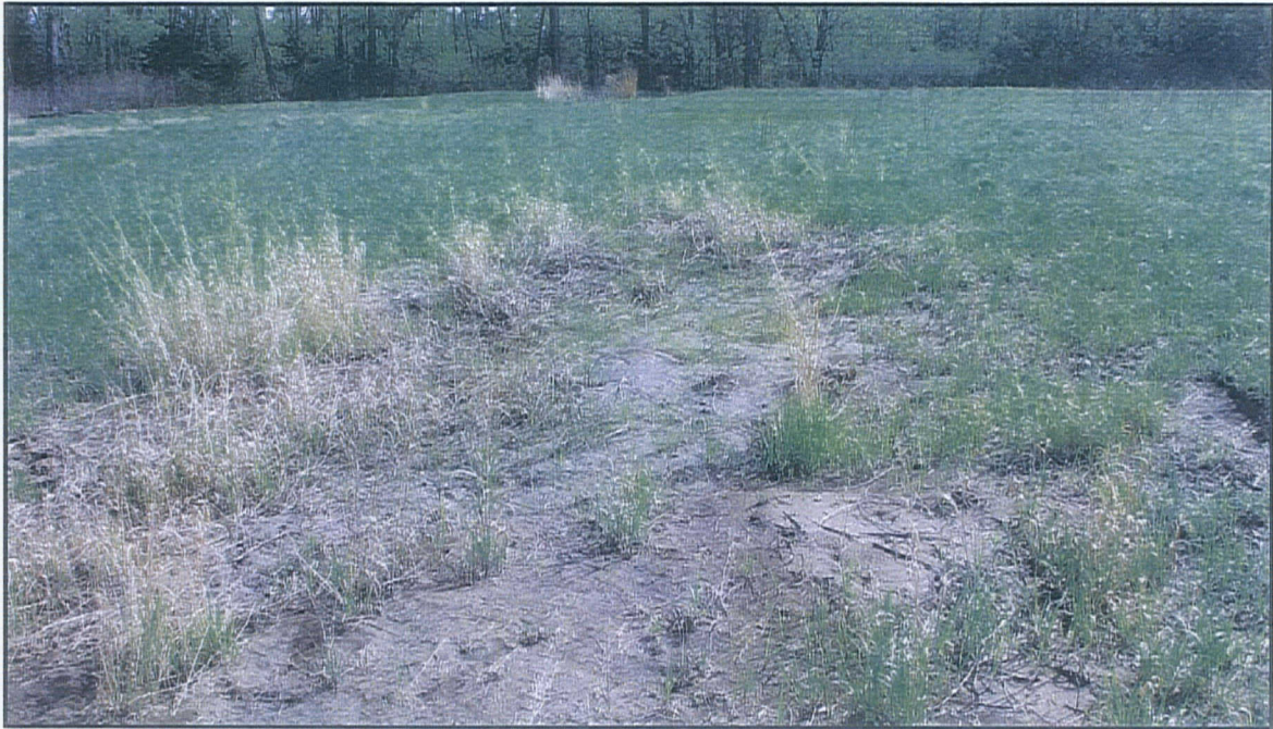
Photograph SFL2009-3 – View looking east at newly repaired area in northeast quadrant of landfill (11 May 09).
