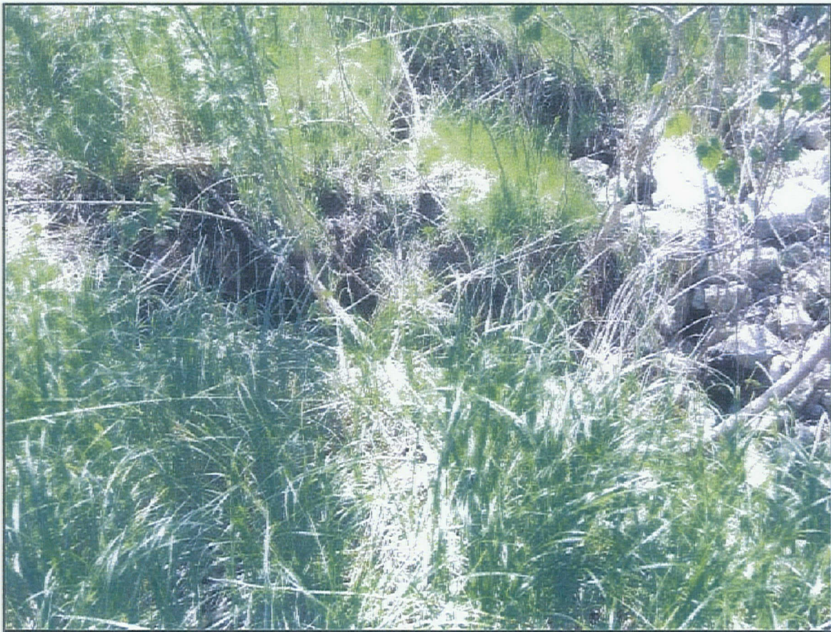
Photograph SFL2009-8 – Back cut erosion at downstream end of revetment (11 May 09).
