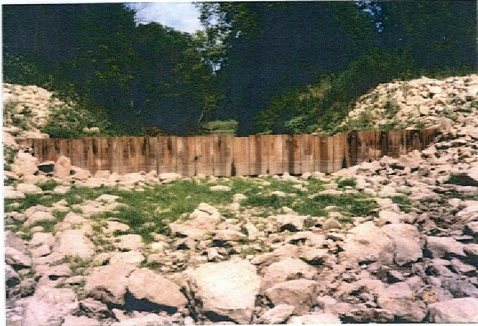
View of sheet pile water diversion structure looking upstream on Threemile Creek (July 30, 1996). The channel bottom and sideslopes are protected with quarry run stone 40 feet upstream and downstream from the water diversion structure.
