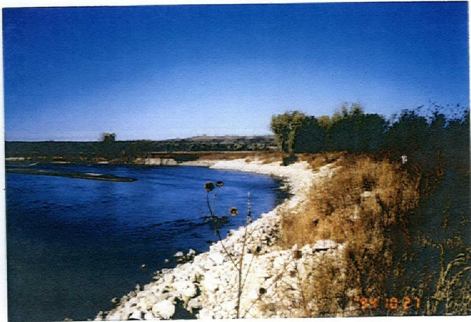
View of Quarry Run Stone Revetment looking upstream (October 27, 1994). The revetment runs parallel to the north bank of the Kansas River and baffles extend perpendicular from revetment to original bank.
