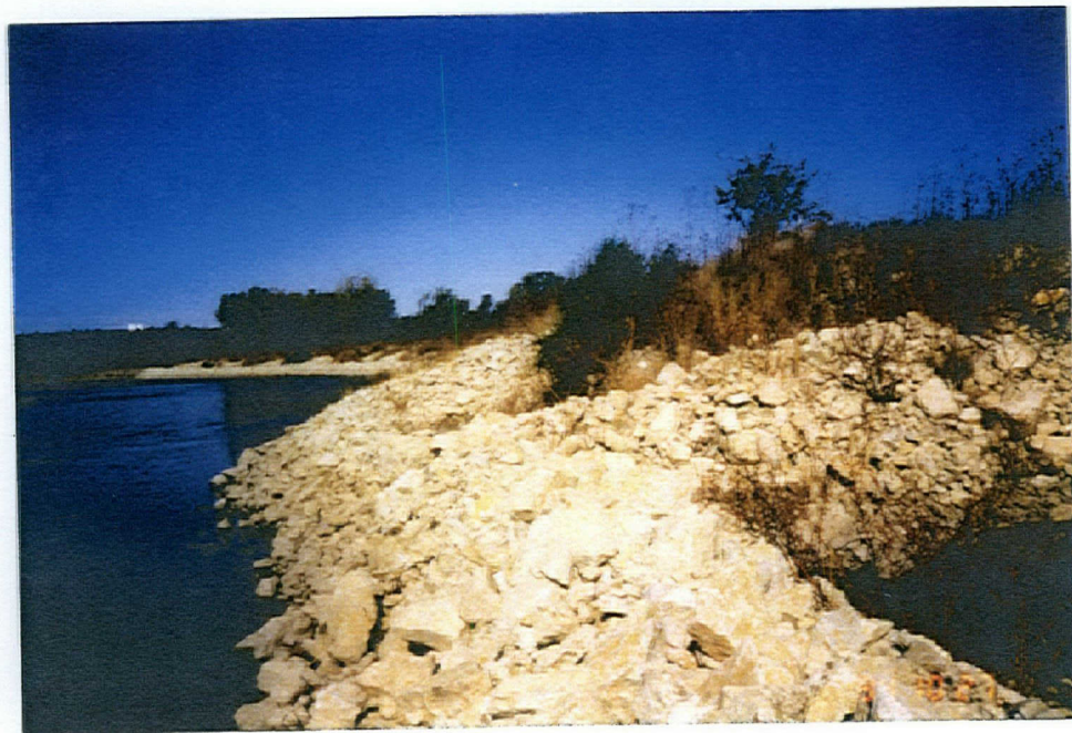
Close-up view (October 27, 1994) of quarry run stone baffle running perpendicular to revetment and original river bank.
