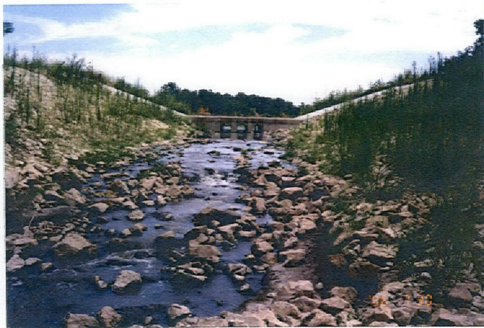
View of concrete water control structure looking upstream in outlet channel (July 30, 1996). The three 30 inch culvert pipe located in the center of structure can be fully or partially closed off with wood baffles to flood the waterfowl management area.
