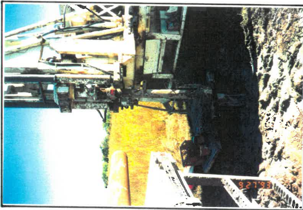
Photograph Number 7 View Toward the Northwest. Mobile B-57 Drill Rig Set Up On OB-93-04
